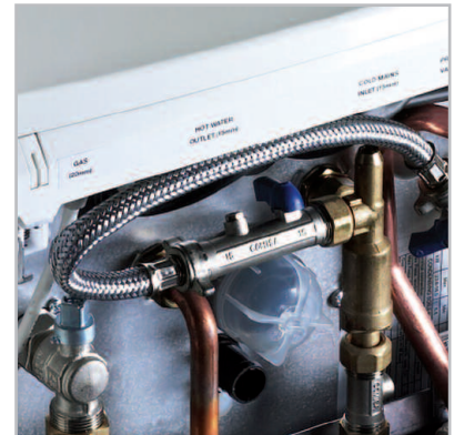
Designed-in filling loop
